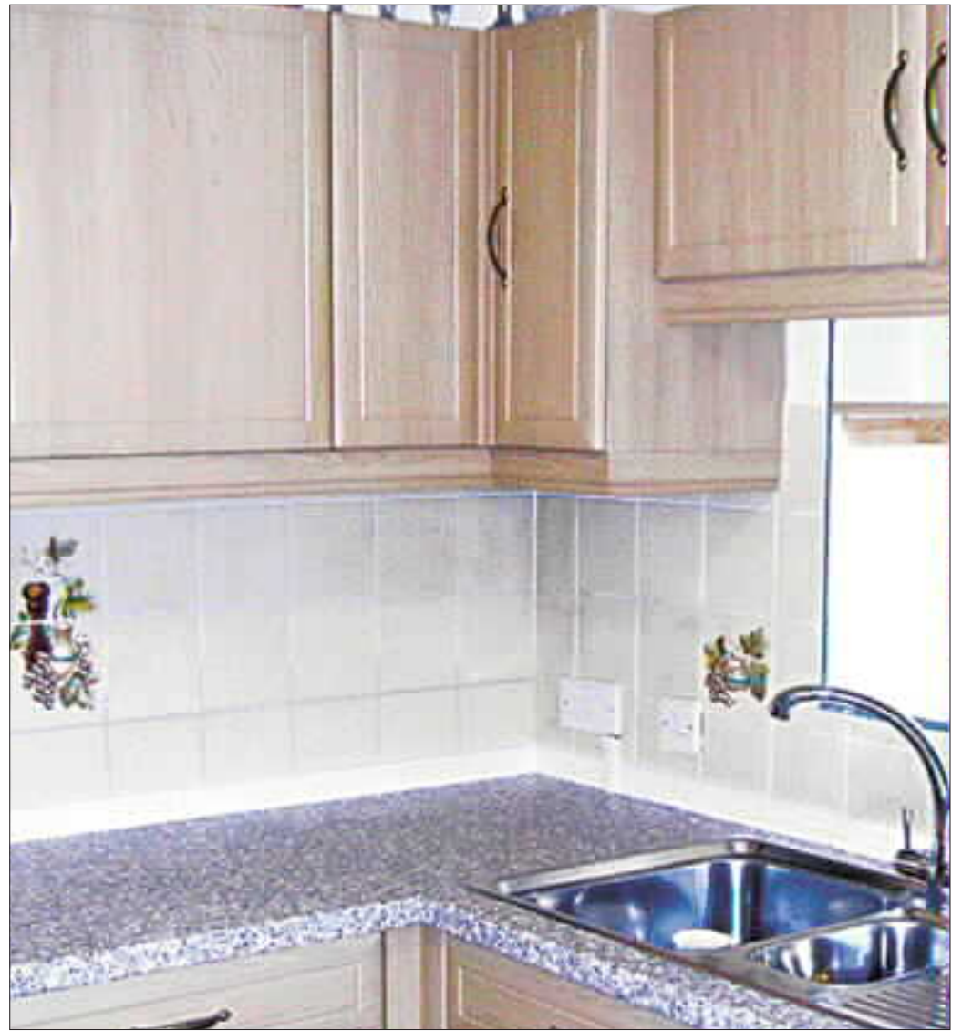
Replacing doors and work tops can breathe new life into your kitchen without huge expense.
